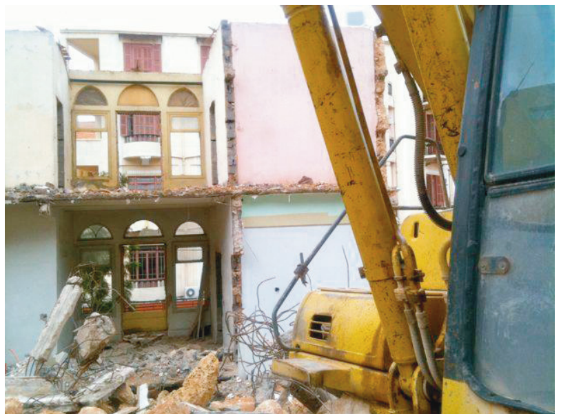
Right: One of the old houses that have been demolished. Only facades were kept.
